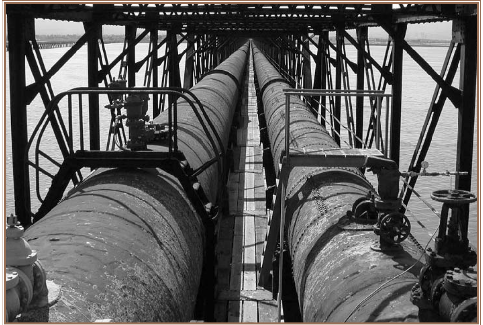
Bay Division Pipelines on trestle bridge
