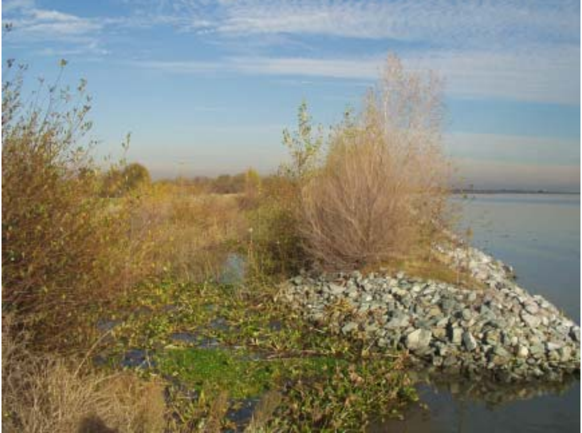
Figure 3. Breach in old levee at Twitchell Island Setback Levee project in spring 2004. Channel between old levee and set back levee is at left. The breach and old levee have been rocked to limit erosion while riparian vegetation takes hold.
