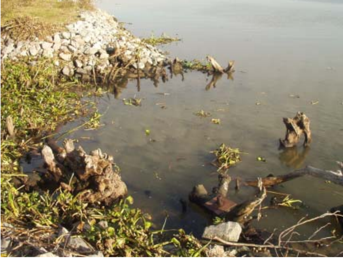
Figure 5. Twitchell project breach with root wads placed for fish cover habitat and erosion control (spring 2004).
