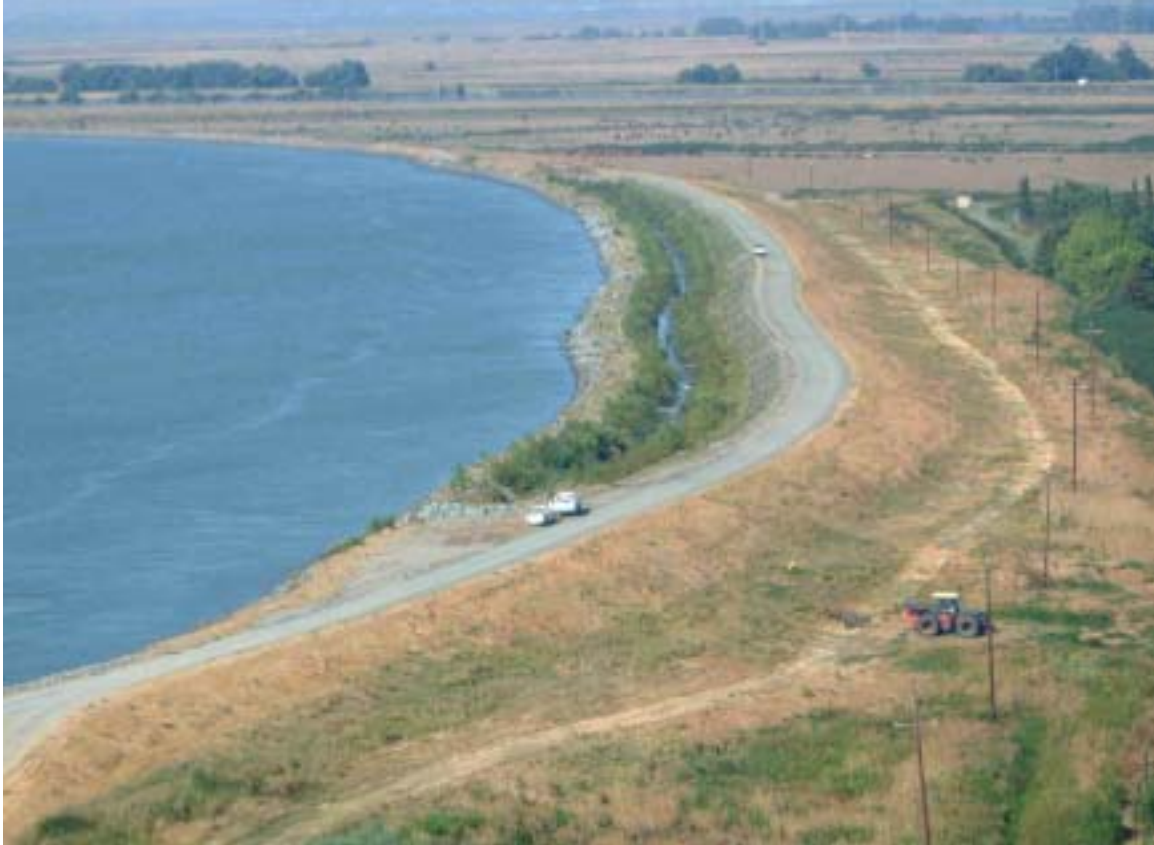
Figure 2. Twitchell Island Setback Levee Project on south shore of Twitchell Island on the lower San Joaquin River channel in the western Delta 2002.
