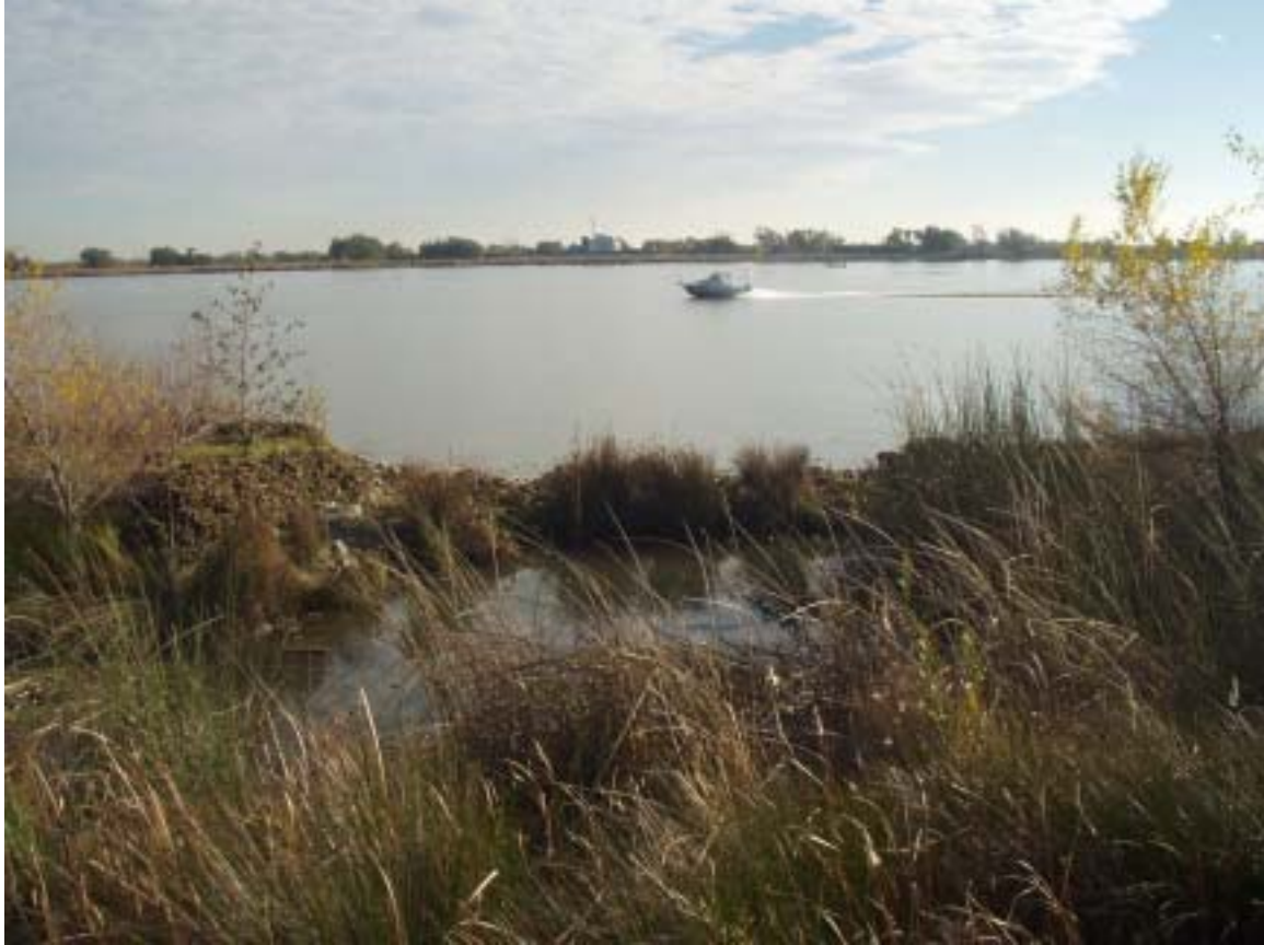
Figure 4. New breaches and habitat are forming where outer levee is eroding (spring 2004).
