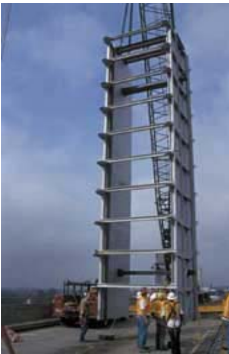
Workers prepare to hoist the Folsom temperature control device into Folsom Reservoir.
