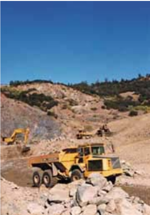
Construction got under way on the American River Pump Station project in October 2003.
