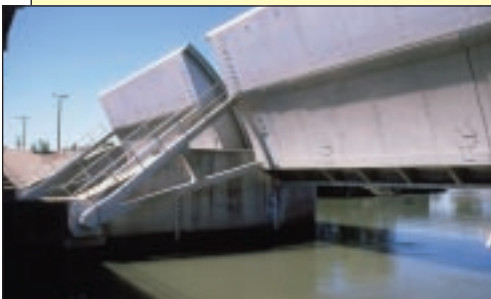
Moveable gates to the Delta Cross Channel. Open, the gates allowed tidal flows of about 9,000 cubic feet per second (cfs) and net flows of about 4,000 cfs to pass through the channel, according to fall 2000 hydrodynamic monitoring.
